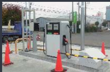
Self-refueling facility installed in Co-op Deli Narashino Center.
